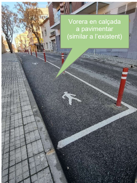
Tram vorera a consolidar
