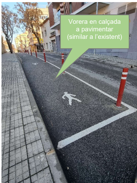
Tram vorera a consolidar
